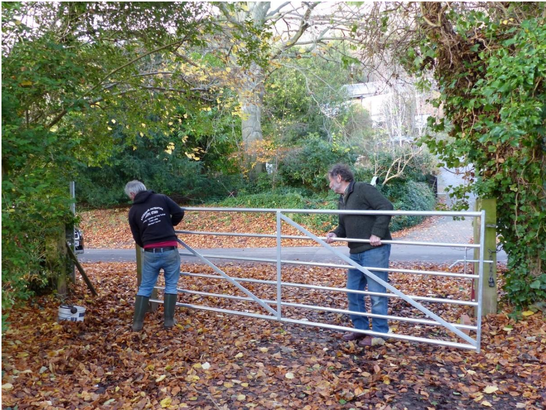
Volunteers Keith Brooks and Pete Woolhouse manoeuvre the new gate into position. They will also be painting it.
