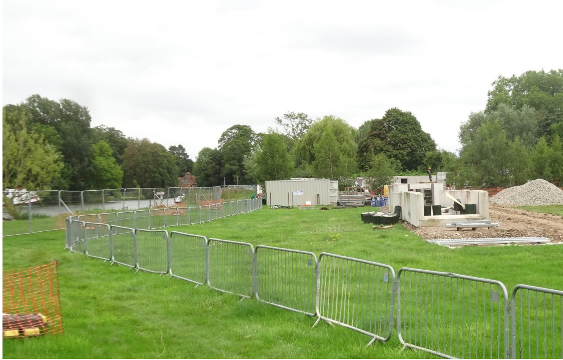
Concrete fish pass units under construction near the riverbank. Mapledurham Mill can be seen in the distance.
