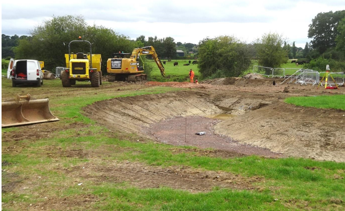
Excavating a channel for the new stream that will convey water from the Thames.
